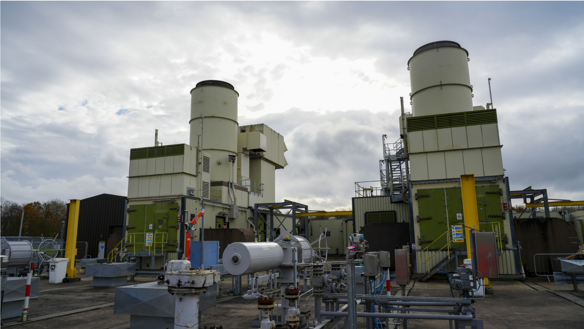
Image 5: Wormington Compressor Station
