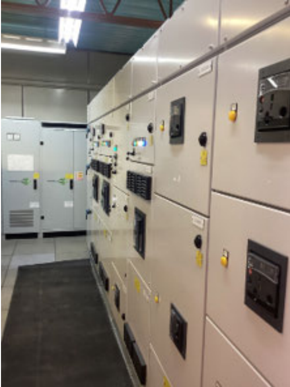
Image 39: LV Switchgear commissioned at [redacted]
