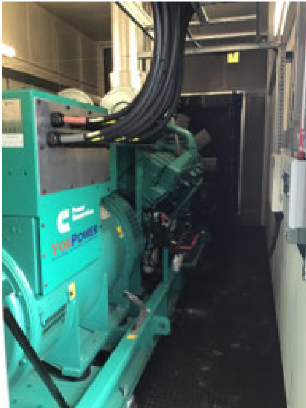
Image 38: [redacted] Standby Generator
