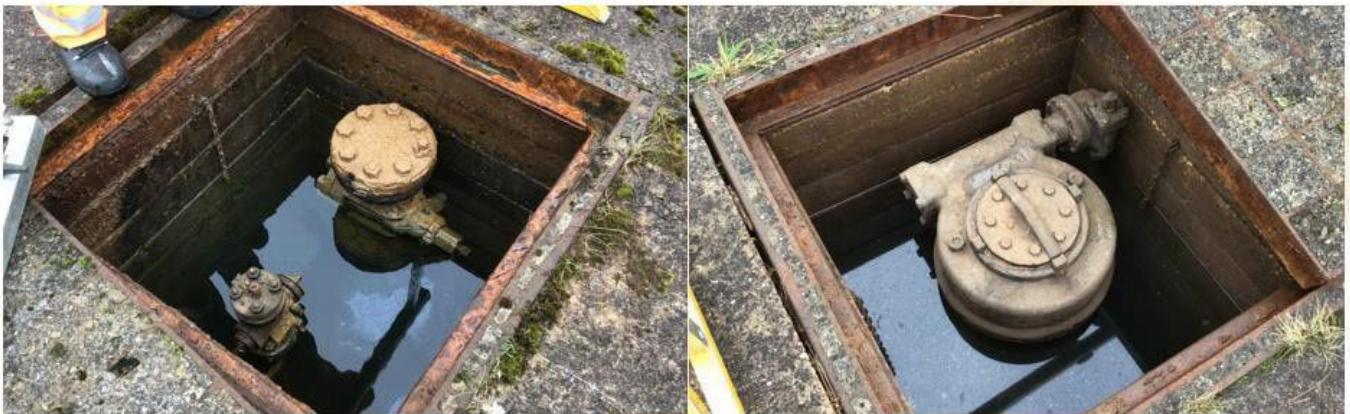
Figure 3: Insufficiently sized pit for valve maintainability
