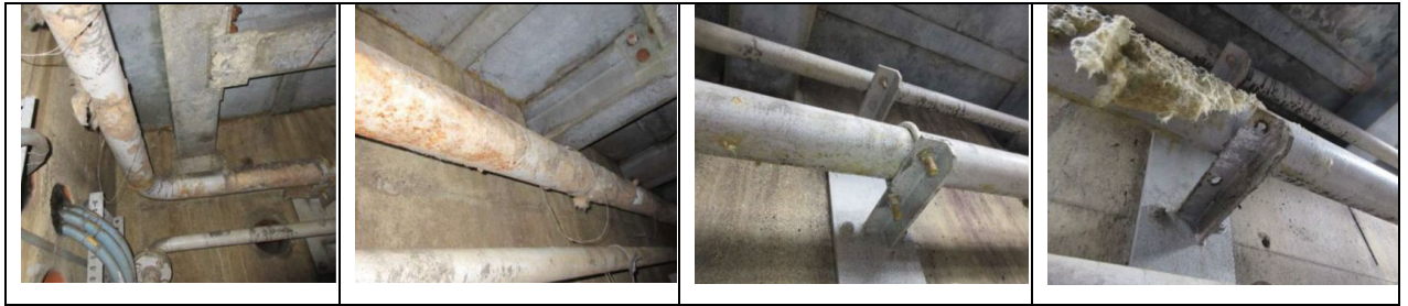
Figure 10: Fuel Gas Inlet Pit
