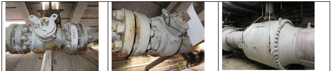
Figure 7: Suction Line Valves
