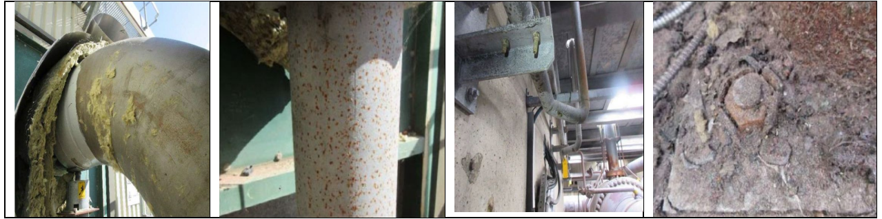
Figure 6: Pipework - Discharge Lines
