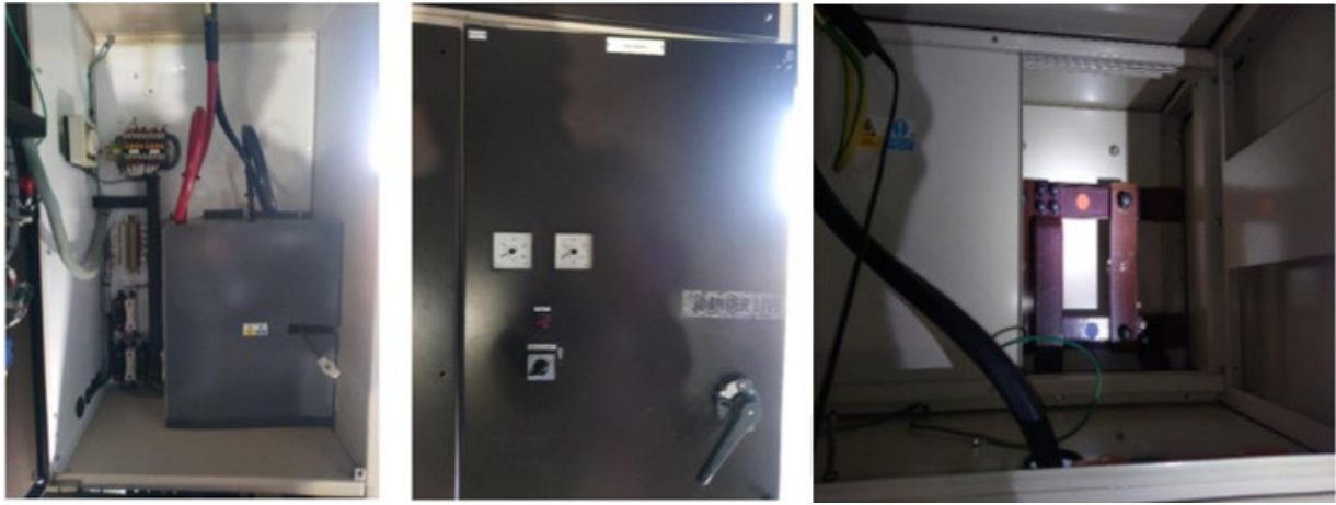
Figure 12: Motor Control Centre
