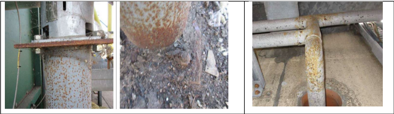
Figure 5: Pipework – Suction Line
