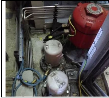
Figure 9: Lube Oil Heater
