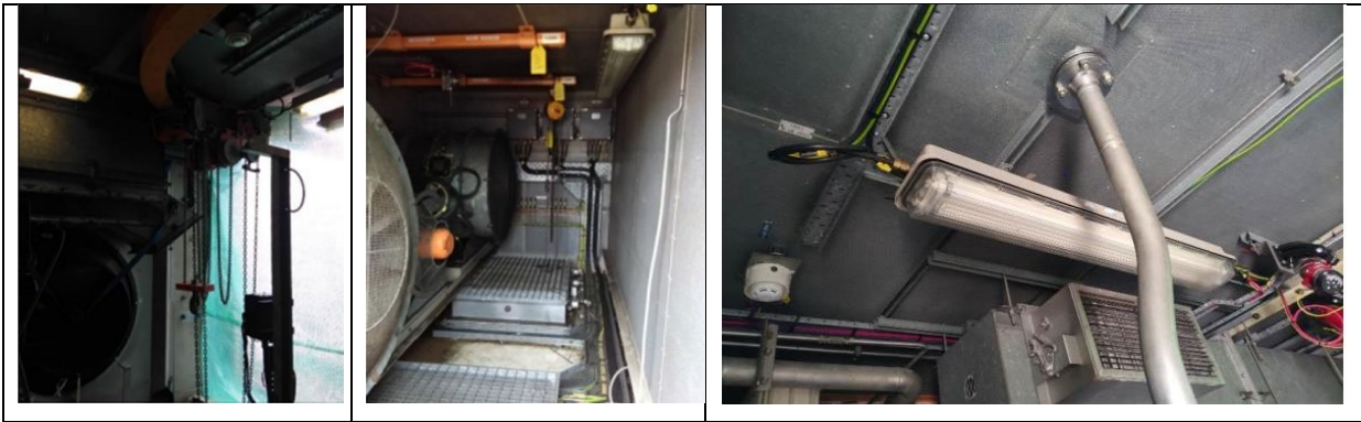
Figure 15: Internal and External CAB Lighting
