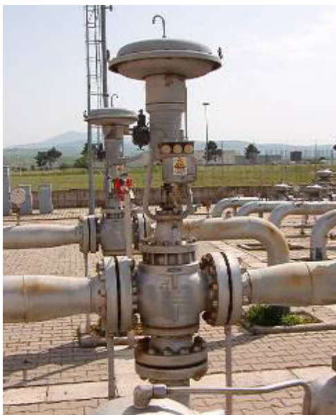
Figure 3.5: Example of a flow control valve
