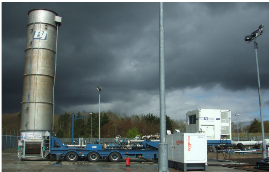
Figure A7.3: Flaring rig
