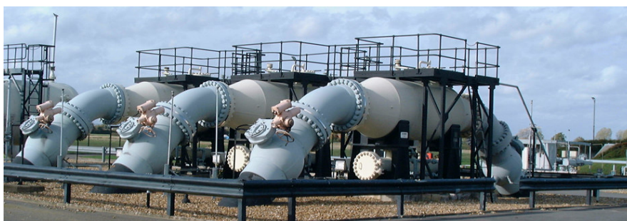
Figure 3.6: Example of a scrubber on the NTS
